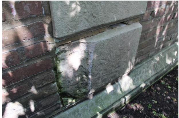
Figure 23. Spalled limestone pilaster on the exterior face of the east courtyard wall.
