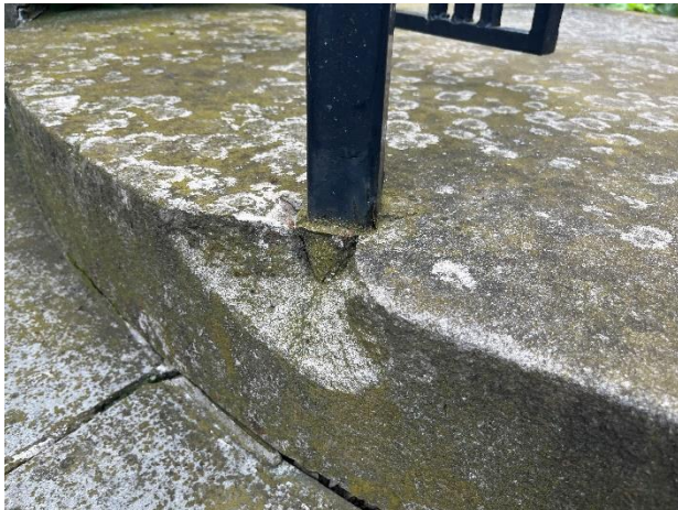
Figure 34. Spalled stair riser.
