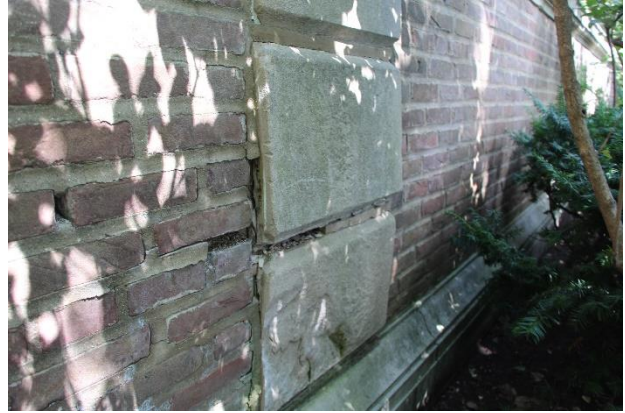
Figure 21. Deteriorated mortar joints.
