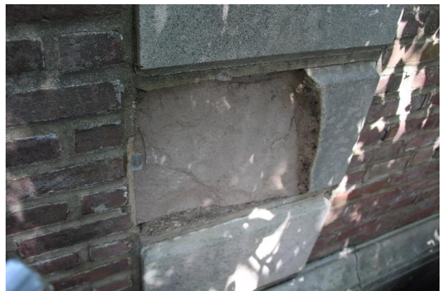
Figure 25. Spalled limestone pilaster on the exterior face of the east courtyard wall.
