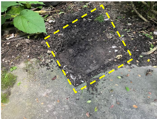
Figure 36. Abandoned clogged drain.
