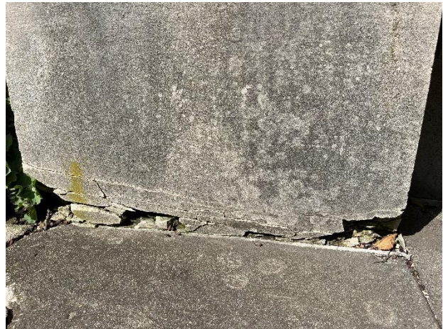
Figure 43. Spalled limestone at the base of a pier.
