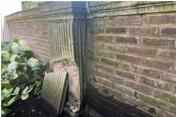
Figure 22. Spalled limestone pilaster in the west courtyard.
