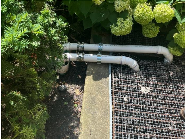
Figure 38. Sump pump discharge piping.
