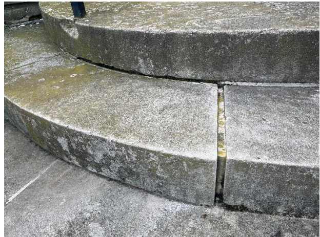
Figure 35. Displaced stair riser.
