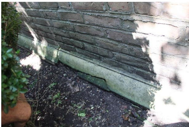
Figure 24. Spalled limestone near grade on the exterior side of the east courtyard wall.
