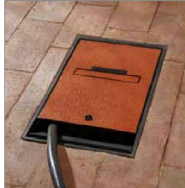
PHOTO 2B: OUTDOOR FLOOR BOX WHILE IN USE
