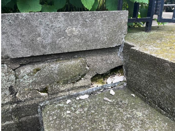
Figure 32. Spalled limestone at the east courtyard east wall.
