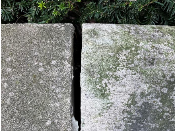
Figure 46. Open joint between bench units.
