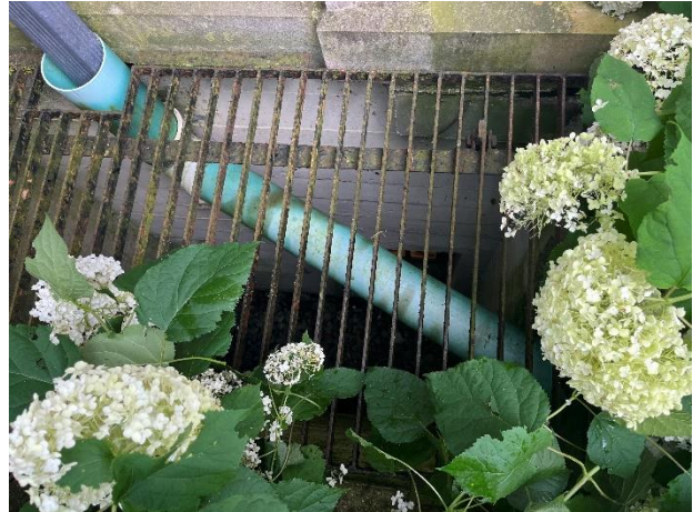
Figure 39. Plastic piping connected to downspout.
