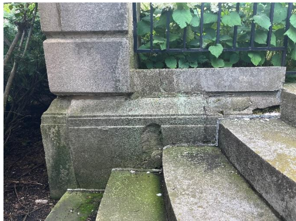
Figure 31. Spalled and cracked limestone at the east courtyard east wall.
