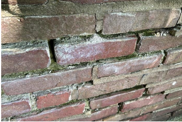
Figure 20. Deteriorated mortar joints and loose bricks.
