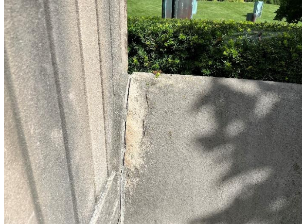
Figure 47. Shallow spall on bench unit where it abuts the pier.
