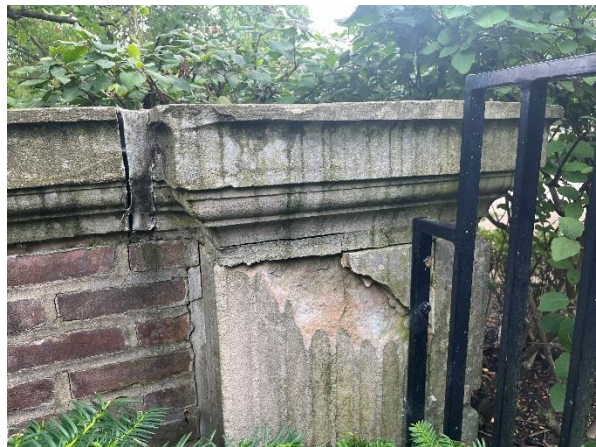
Figure 29. Damaged limestone related to movement of the non-original steel fence.
