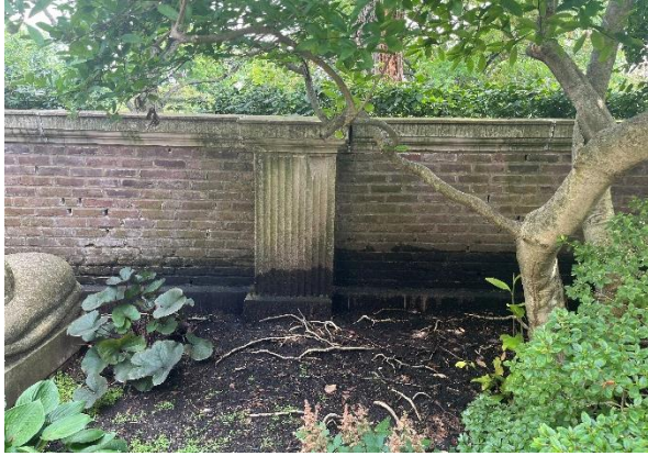
Figure 26. Staining near grade on the courtyard wall.
