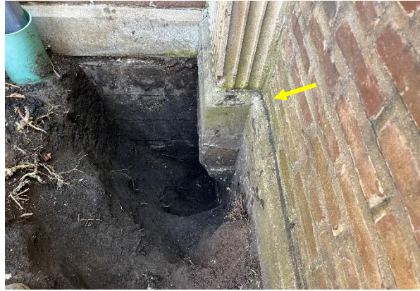
Figure 27. The concrete structure extends above grade on the interior face of the courtyard wall (to the joint marked by the arrow).
