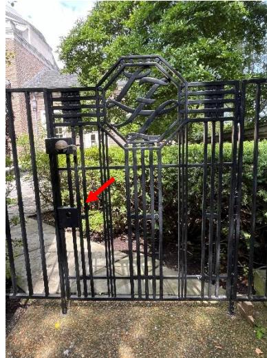
Figure 6. Existing appearance of the gate. When the masonry walls were lowered in height, the gates were trimmed at the top and bottom to fit the altered opening. The latch handle was relocated to a new location; the arrow indicates the original latch box.
