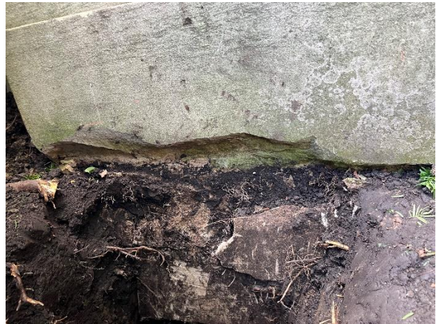
Figure 45. Spalled limestone at the base of a pier.
