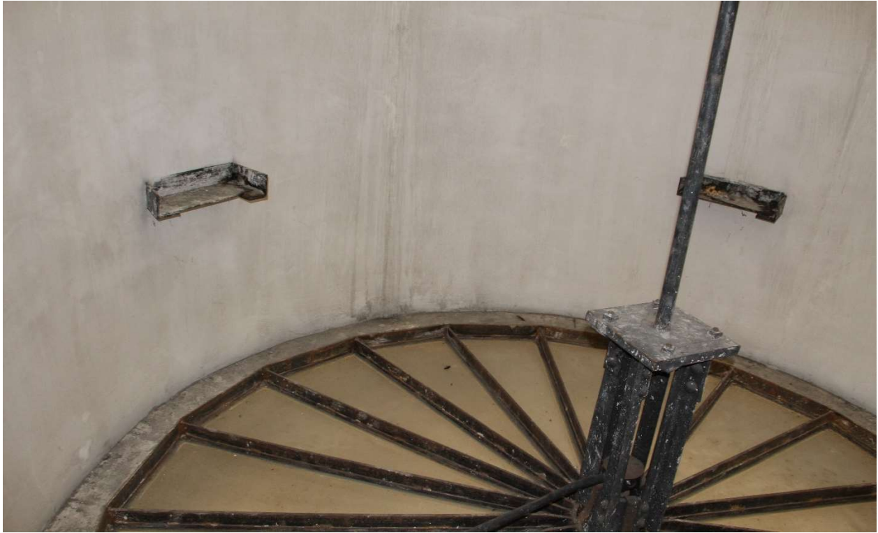
Figure 1. Wall brackets and central hub above laylight.
