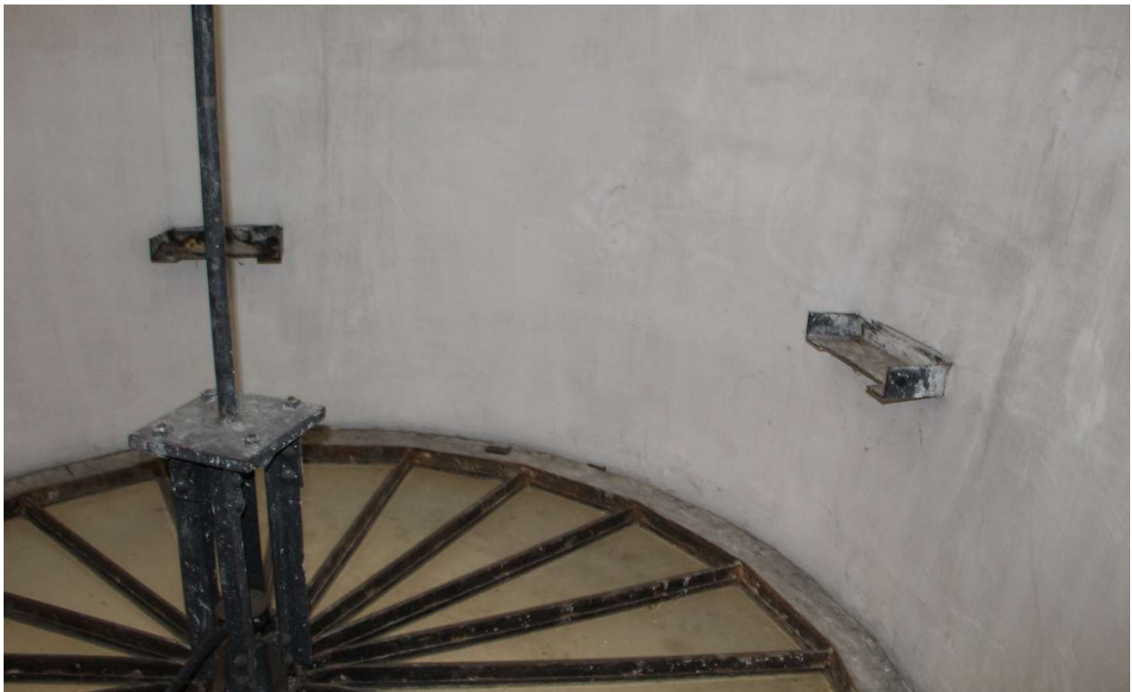
Figure 2. Wall brackets and central hub above laylight.
